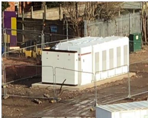
Tesla 2.1MWh Battery - 500kW inverter
