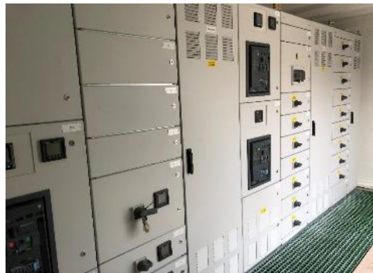
Low Voltage Distribution Panels
