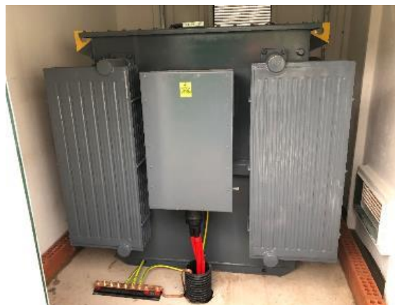
Energy Centre Sub Station
